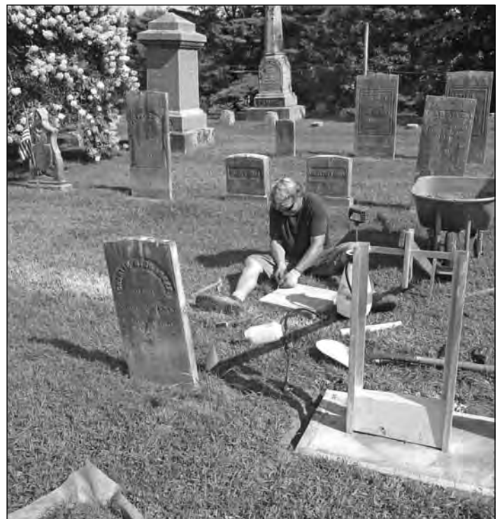
Standing Stone repairing cemetery stones in the old section of Fairlee Village Cemetery.
